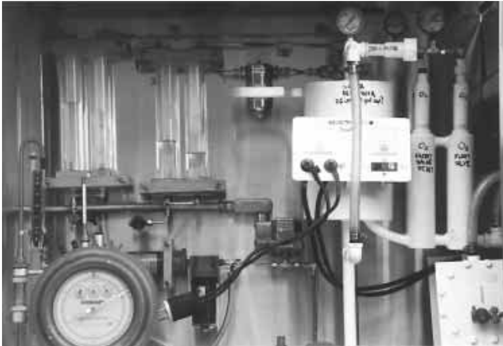
Above: The bi-directional bubblers and purification systems. Photo by Reynaldo Cortez
